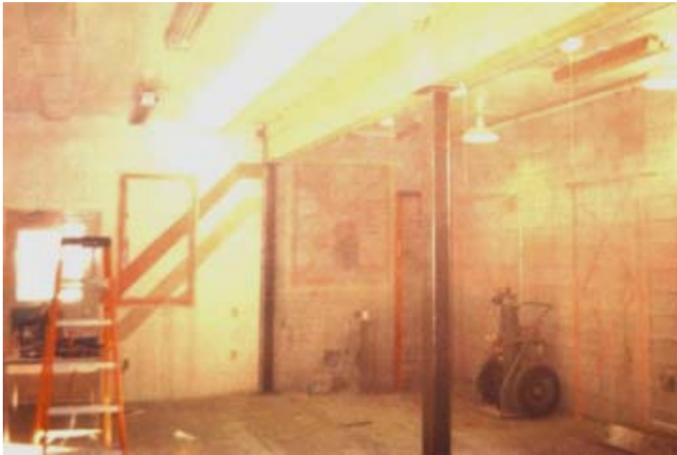
Figure 7. Southeast wall prior to cement cutting to access outside entrance restrooms (on right).
